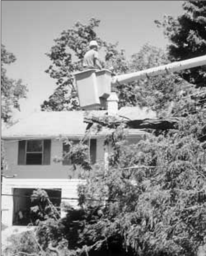
Foreman Chad Behnke has a real job ahead of him clearing the limbs from these power lines.
