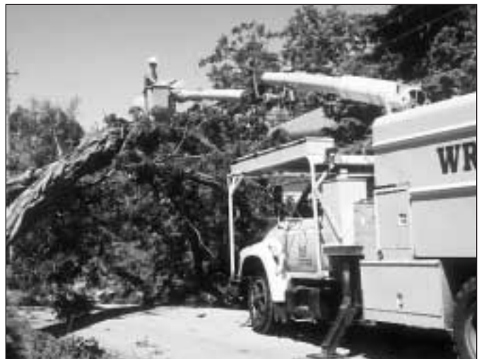
This fallen tree formed an arch across the road. Foreman Chad Behnke is in the bucket.
