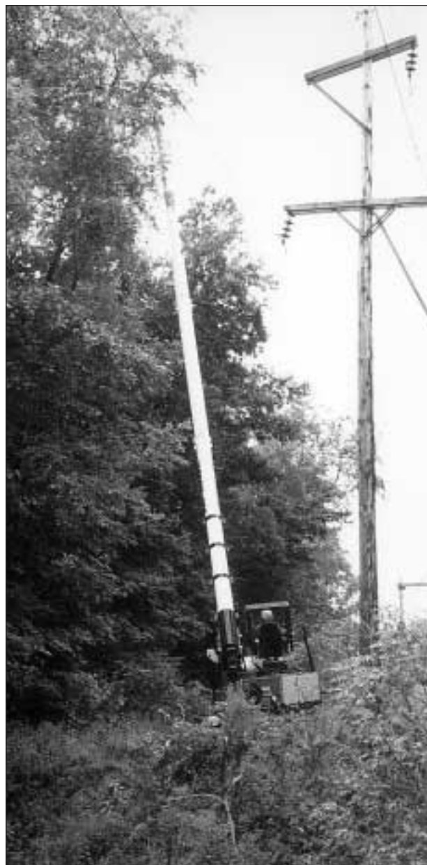
With the boom extended to its maximum height, the Jarraff Tree Climber is ready to take on limbs 75 feet high.
